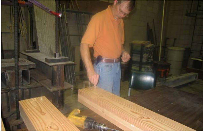
Figure 6.21. Assembly of the Glulam Specimens with Non-Structural Packages: Insertion of the Wooden Dowels
