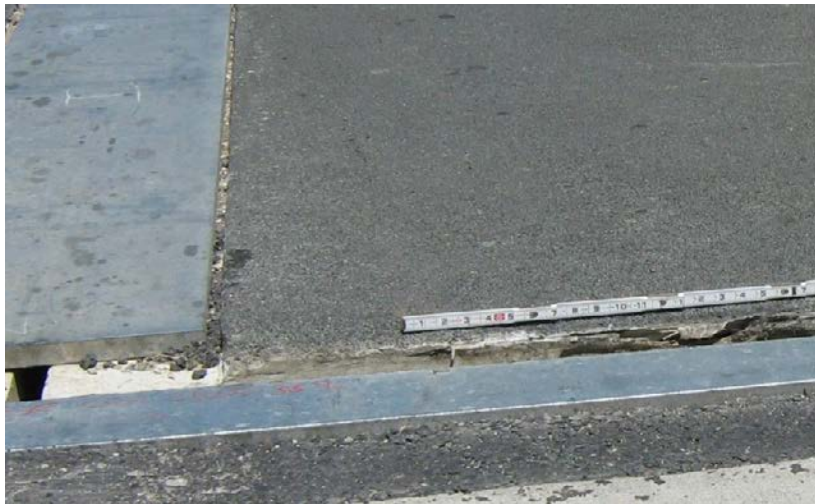
(b) Deterioration at end of deck panel
